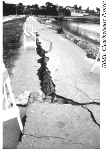
Figure 39 - Lateral Spreading. Loma Prieta Earthquake, October 17, 1989. Lateral spreading damage levee road along the San Lorenzo River.
